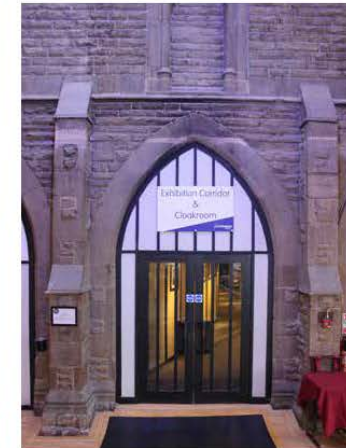
View of the wall between the 1967's Foyer and the Main House
