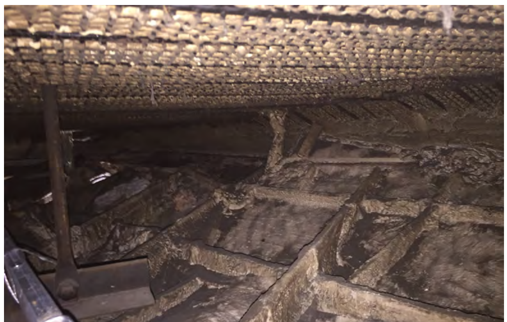
Figure 29: Large area of ceiling installed without sufficient wad connections to the panels. This can be easily detected in an inspection and remedied in subsequent repairs.
