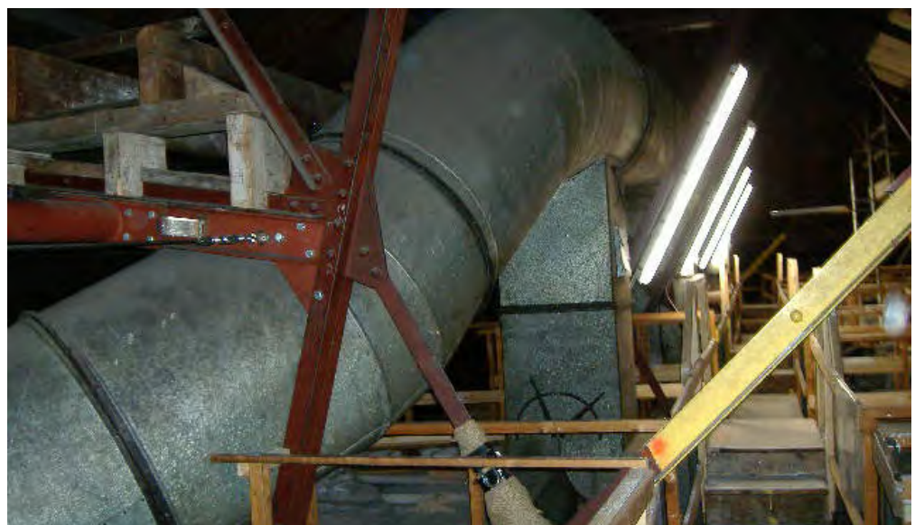
Figure 31: In ceiling voids bulky mechanical plant and boarded walkways (lower right) obscure the fibrous plaster ceiling below and impede its inspection.
