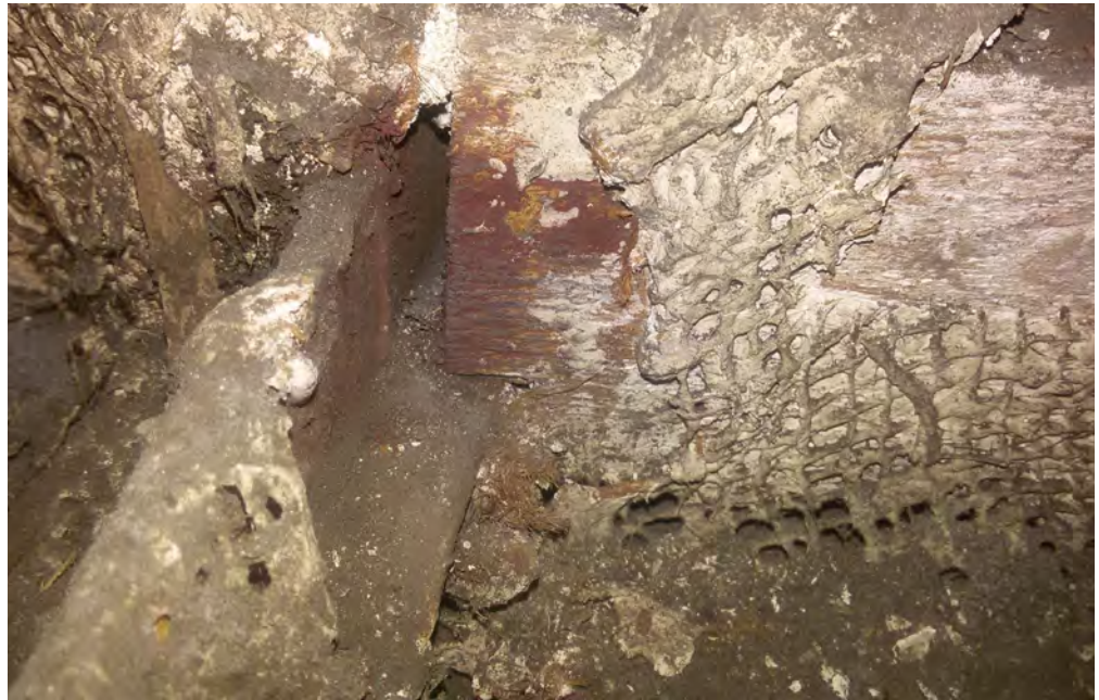
Figure 30: Poor bearing of a timber ceiling joist on a small steel T bar. The hessian has insufficient plaster cover to protect it from degradation. This illustrates how defects can be concentrated.
